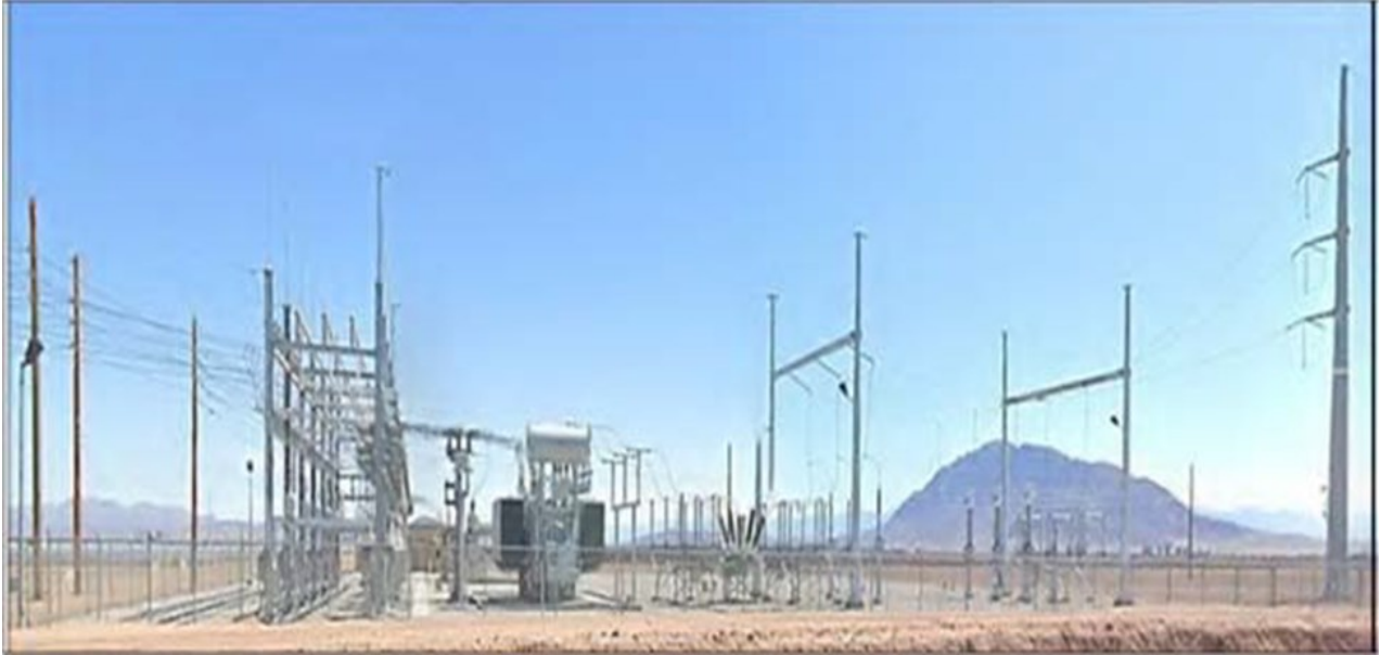
Photo PD-2: Proposed Project Conceptual 230 kV Substation.
