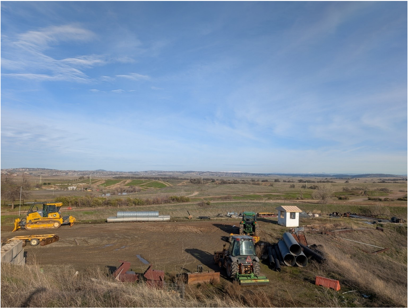
KOP 9i. Looking East/Northeast from the Prairie City SVRA Picnic Area/Overlook. A construction staging yard containing heavy construction equipment, metal piping and other miscellaneous objects is visible in the foreground and midground. Grasslands, scattered trees, buildings, and the rolling hills of the Sierra Nevada are visible in the background.
