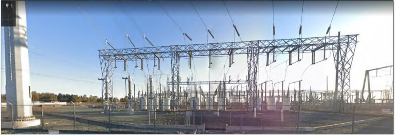
Exhibit 1A. Gen-tie line of similar 230 kV switchyard in Sacramento County.
