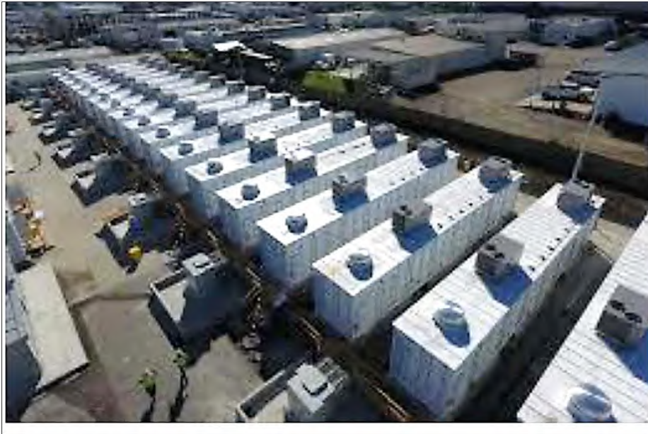
Exhibit 3A. Examples of battery storage containers.
