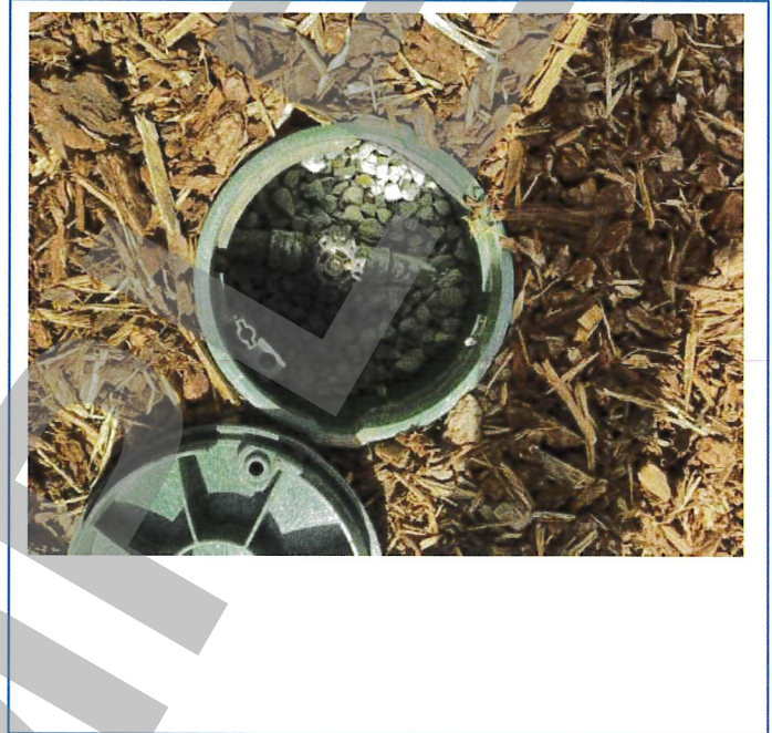
Irrigation Shut Off Valve
