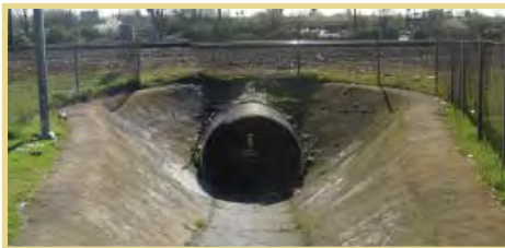
The pedestrian underpass near Watt Avenue and Roseville Road is subject to a feasibility study to determine possible improvements.
